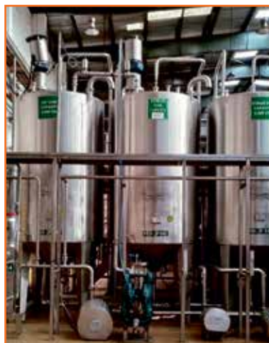
Fig 5.2.3 Storage Tank for Ketchup Making
